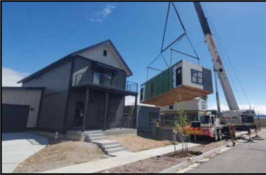
A second mod is lowered by crane onto an already set mod, completing this home's second story. The home is located in Quartz at Poncha Meadows, Poncha Springs, Colorado.
