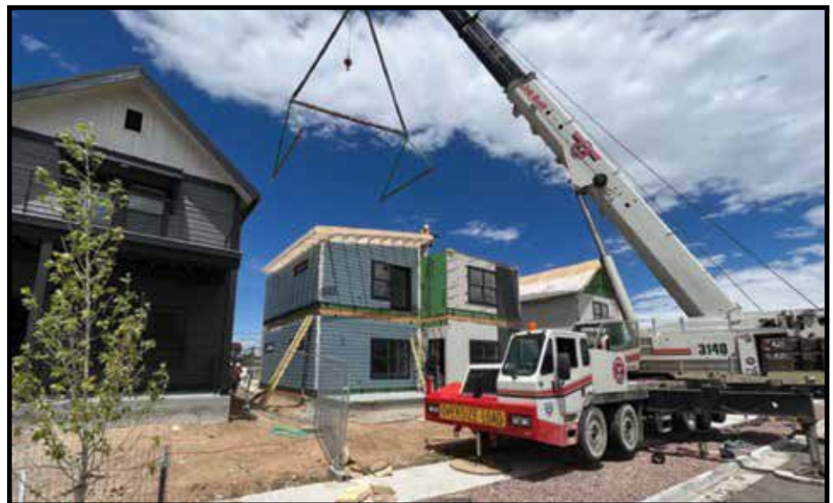
The roof and other final elements are completed on-site once the modular home is set. Located in Quartz at Poncha Meadows, Poncha Springs, Colorado.
